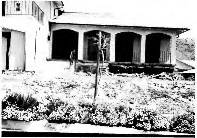
Photo 24. Note tilting and partial collapse of vertical bracings (cripples, lower right portion of structure) between floor and footing wall which allowed single-story unit to settle and move away from two-story unit.
